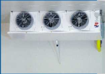
The Güntner Vario CUBIC GHN air coolers installed in the cold storage have only a low temperature difference between supply air and exhaust air. This operating mode is chosen to avoid losses of weight of the raw vegetables and fruits caused by evaporation.
