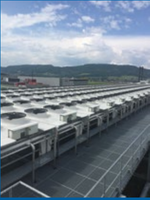
▲ 27 AGVH-type Güntner FLAT Vario condensers are used to dissipate the heat that cannot be used in production from four central ammonia refrigeration circuits in the combined bakery/deep-freeze storage building.
