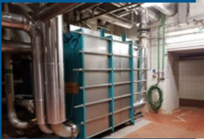
▲ In Tychy, wort is cooled from 99 °C to 10 °C using five thermowave TL 500 TCGL plate heat exchangers with a combined plate heat exchanger capacity of 32 MW.
