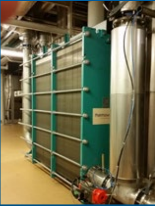
▲ A thermowave TL 850 KBKL unit with a heat exchanger capacity of 6.5 MW heats up over 200 m 3 of wort per hour from 72 °C to 98 °C. In the counterflow, 100 °C hot water is cooled as part of this process step down to 78 °C.
