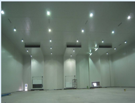
Cold store with channels for refrigeration at -25 °C
