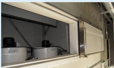
Floor-mounted coolers outside the cold store
